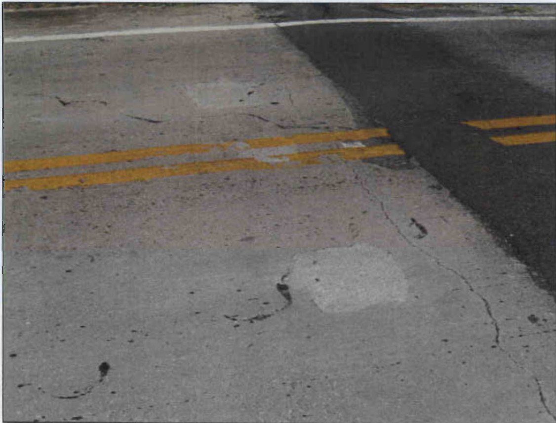
PATCHED AREAS IN SPAN 1 DECK OVER END BENT 1
