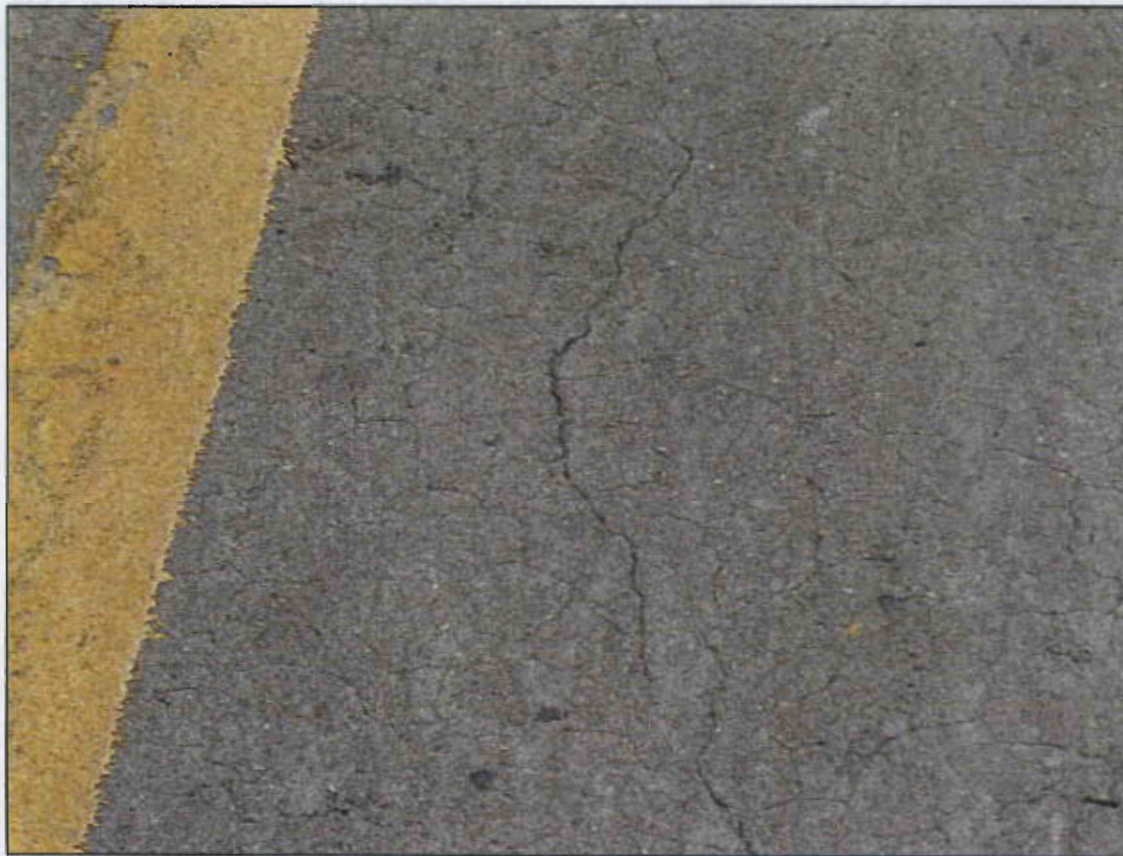
LONGITUDINAL CRACKING IN SPAN 2 DECK UP TO .013" WIDE
