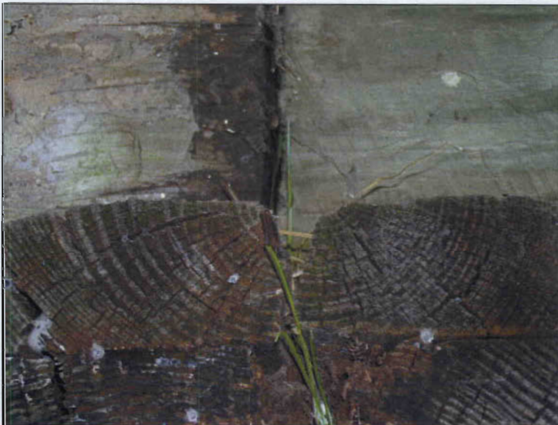
BENT 1 CROWNSTRIP AT SOUTH END DECAYED 1" WIDE X 20" LONG.
