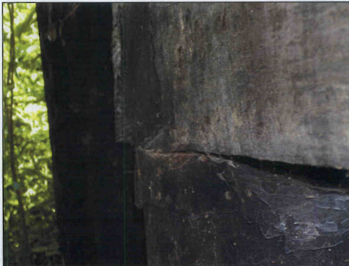
PILE 1 AT END BENT 2 PUSHED OUT 1" DUE TO BULKHEAD PRESSURE (PRIORITY MAINTENANCE)
