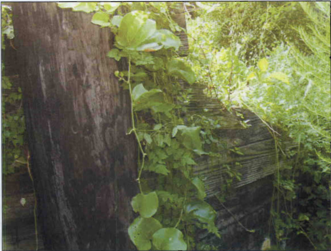
SOUTHEAST EXTERIOR BULKHEAD/WINGWALL DECAYED AND DISPLACED BOARDS
