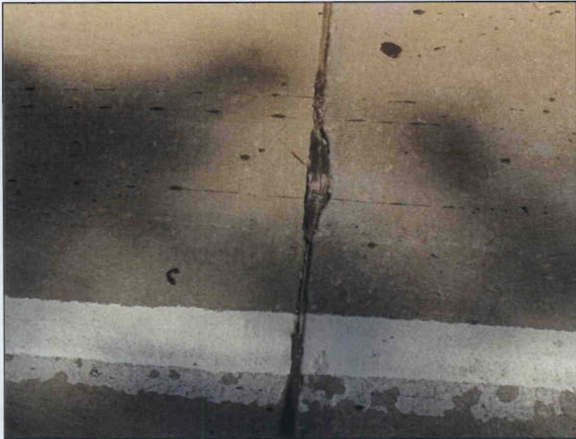
BENT 2 JOINT MATERIAL MISSING AND LOOSE IN A 2' LONG AREA.
