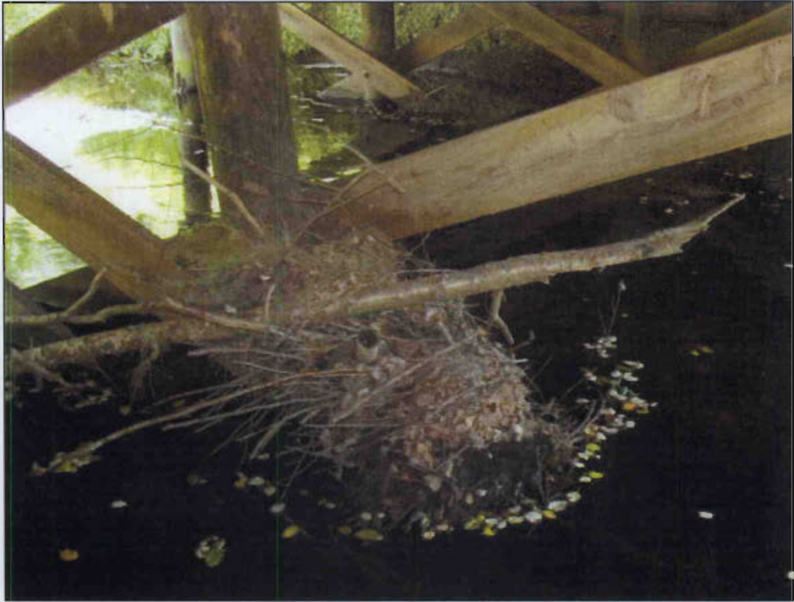
DRIFT COLLECTING AT PILE 3 OF BENT 1
