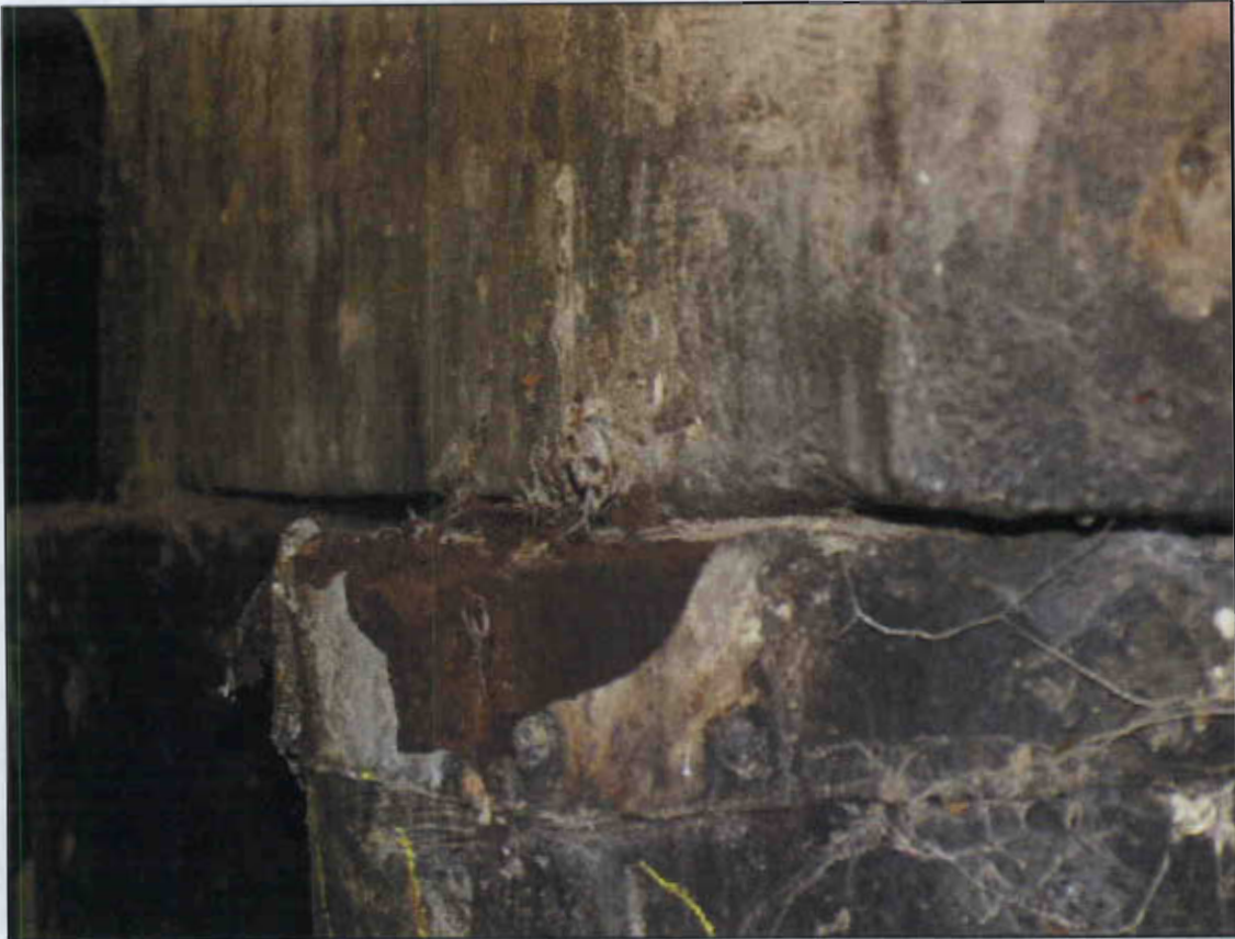
PILE 3 AT END BENT 2 PUSHED OUT 3" DUE TO BULKHEAD PRESSURE. (PRIORITY MAINTENANCE)
