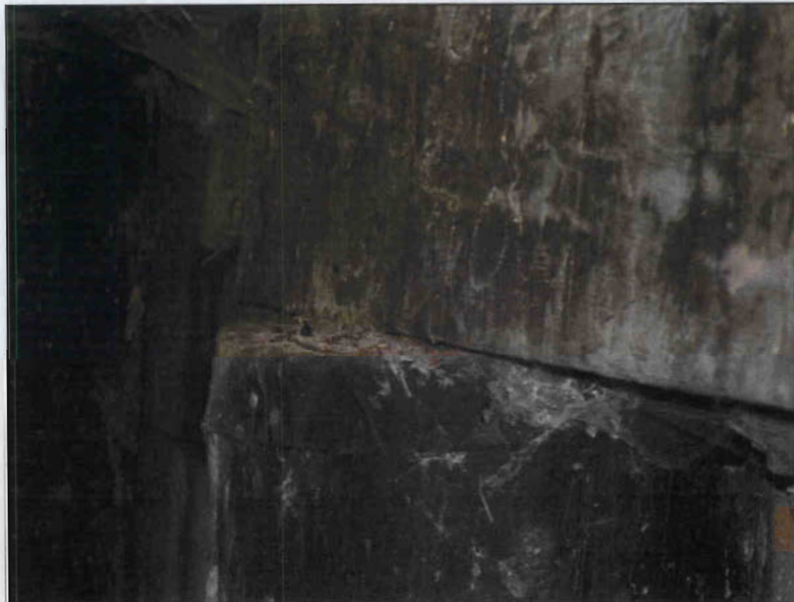
PILE 2 AT END BENT 2 PUSHED OUT 3" DUE TO BULKHEAD PRESSURE.(PRIORITY MAINTENANCE)
