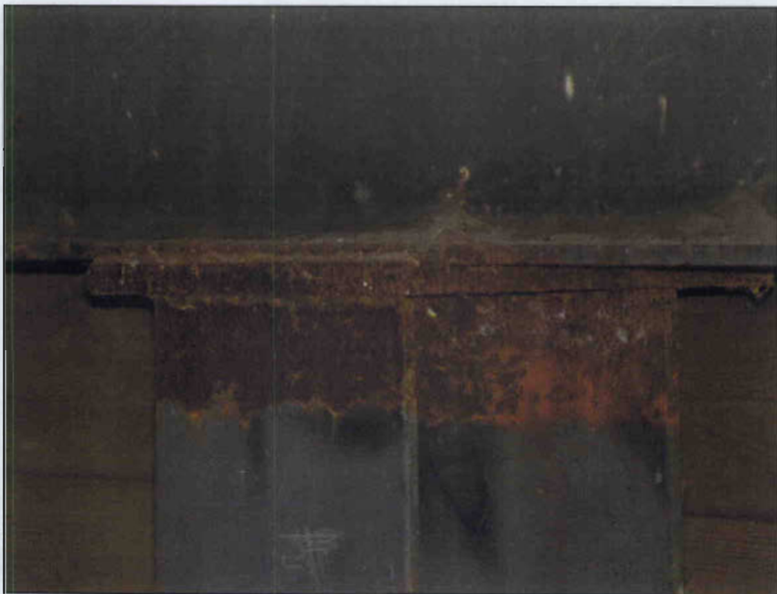
PAINT PEELING WITH SURFACE RUST ON TOP PORTION OF STEEL PILES AT END BENT 1
