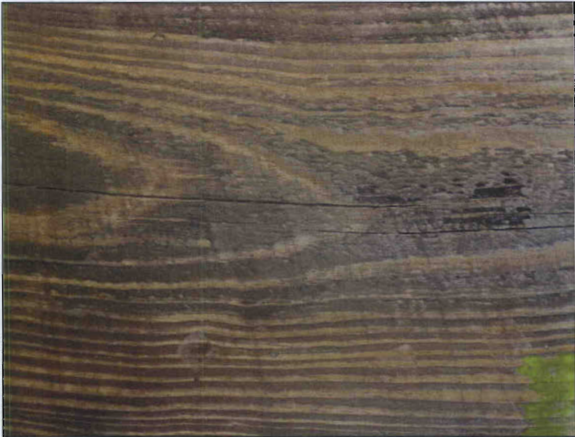
LONGITUDINAL CRACKING ALONG CAPS UP TO 1/8" WIDE
