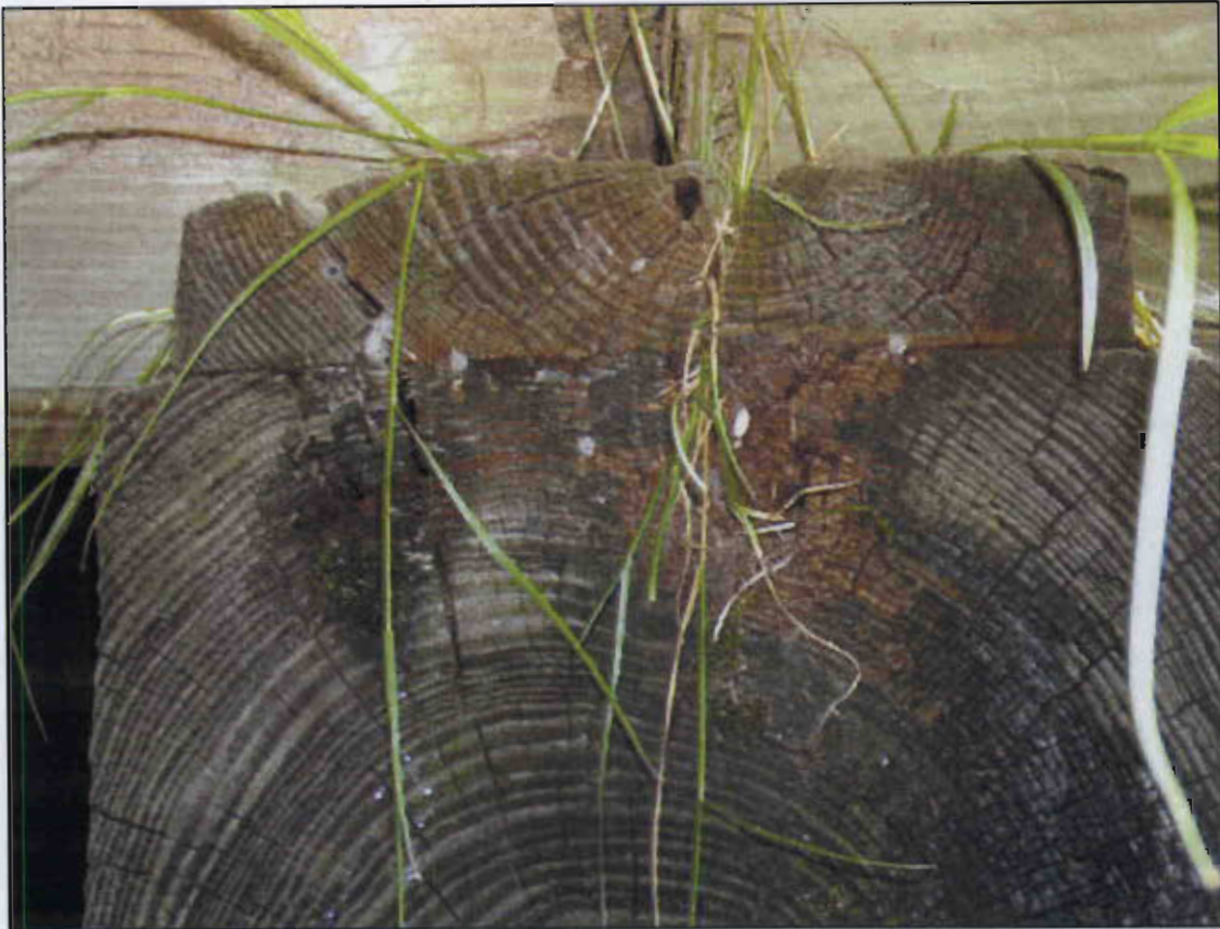
BENT 1 CAP AT SOUTH END 2 DECAYED AREAS 2" DIA. X 6" DEEP
