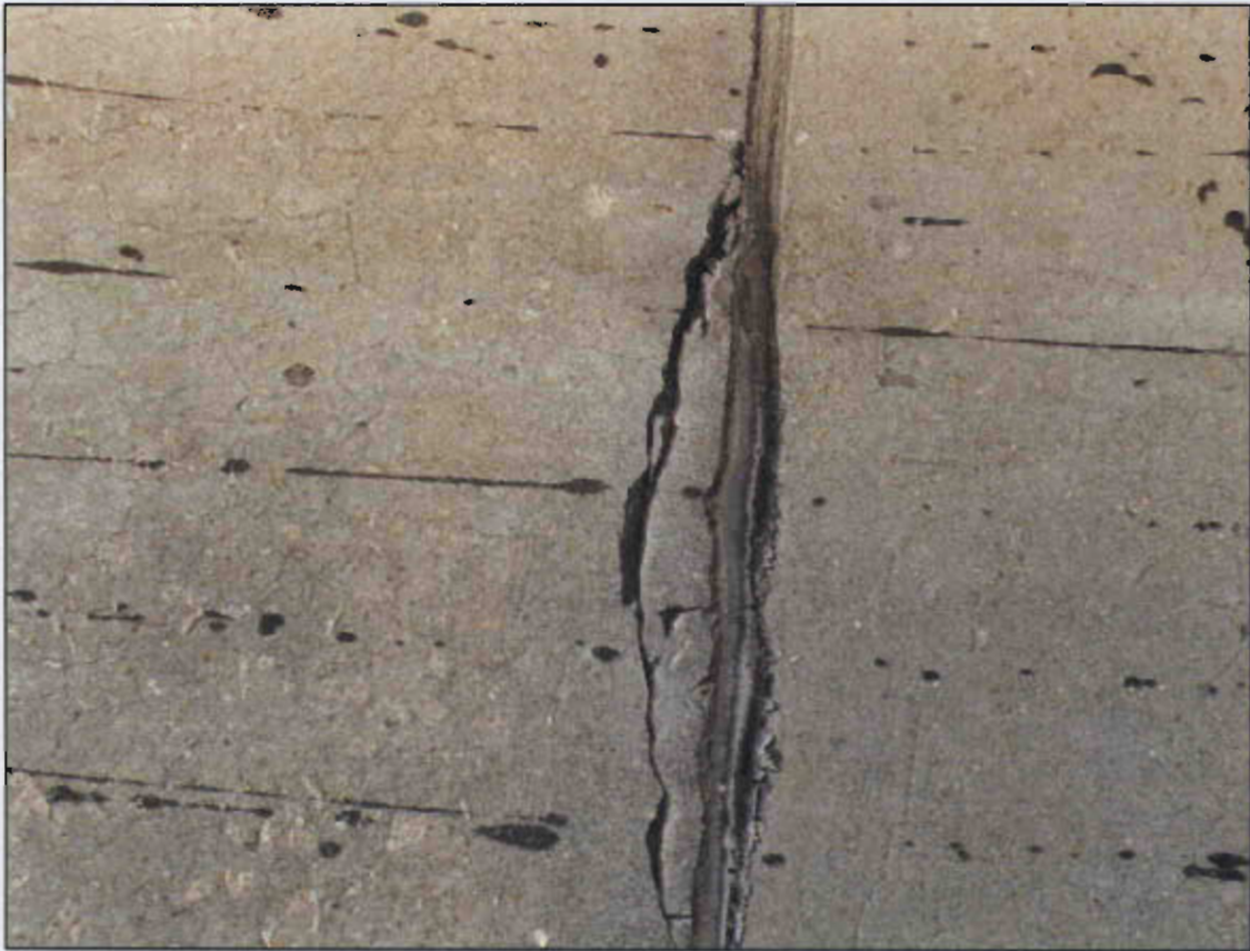
SPAN 3 DECK CRACKED AND DELAMINATED AREA ALONG BENT 2 JOINT IN WEST BOUND LANE 18" LONG X 2" WIDE.
