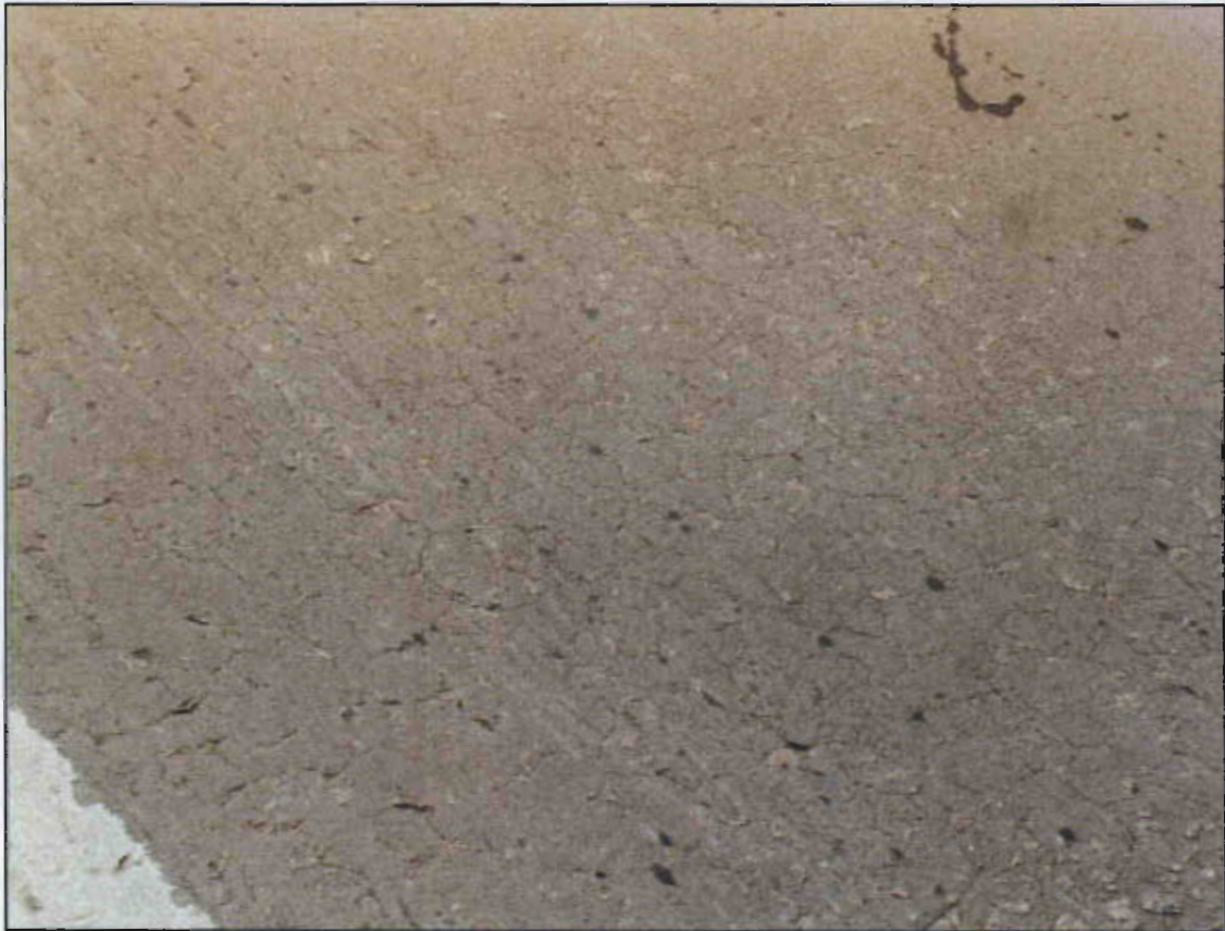
HAIRLINE MAPCRACKING IN DECK IN ALL SPANS
