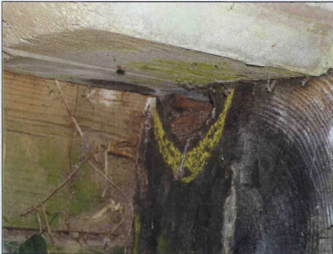
NORTH END OF END BENT 2 CAP DECAYED 12" LONG X 4" WIDE X 2" HIGH
