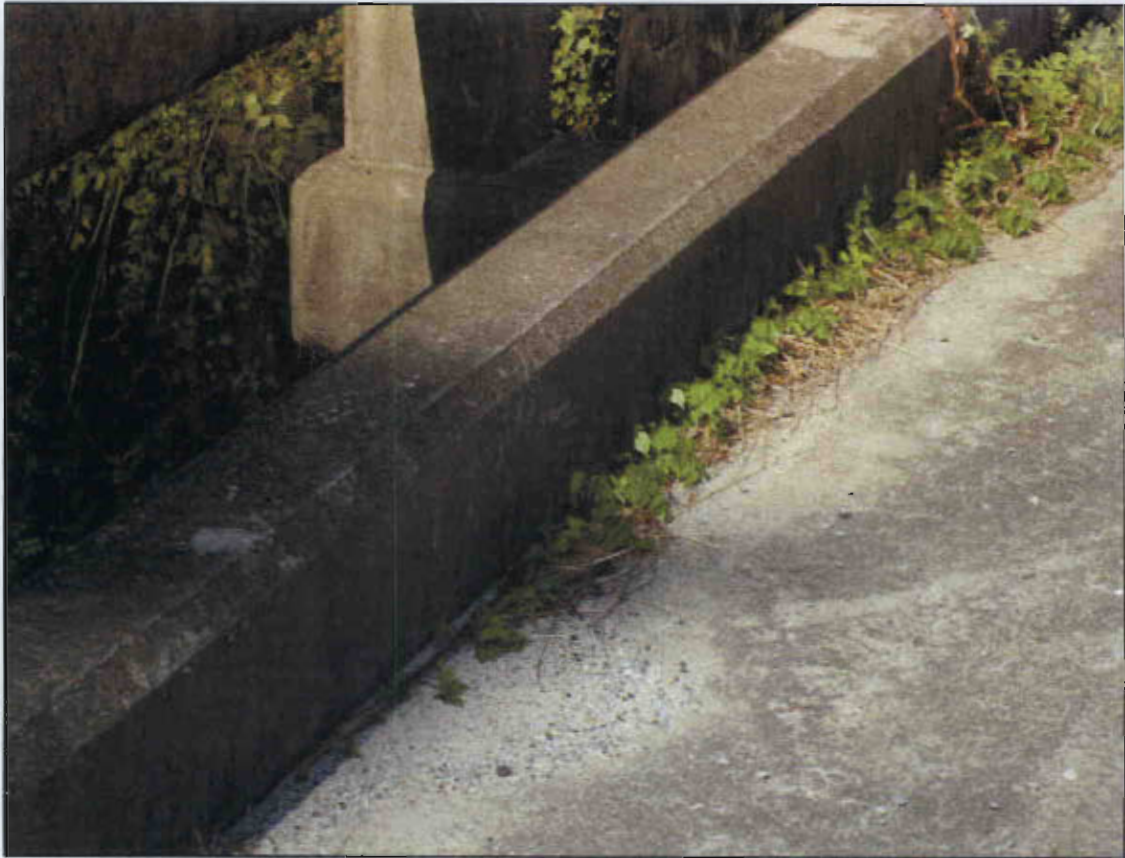
GROWTH AND DEBRIS ALONG SOUTH CURB IN SPAN 1
