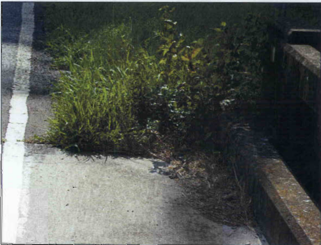
GROWTH AND DEBRIS BUILDUP AT CORNERS OF BRIDGE
