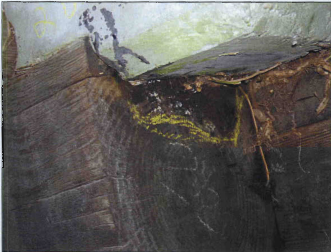
SOUTH END OF END BENT 2 CAP DECAYED 10" WIDE X 3" HIGH X 2" DEEP.
