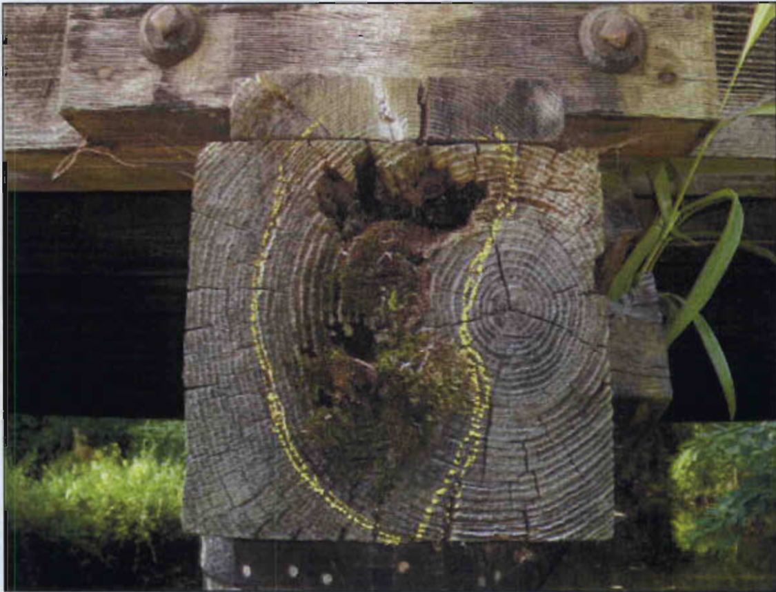
NORTH END OF BENT 1 CAP DECAYED 5" WIDE X 10" HIGH X 12" DEEP.(PRIORITY MAINTENANCE)
