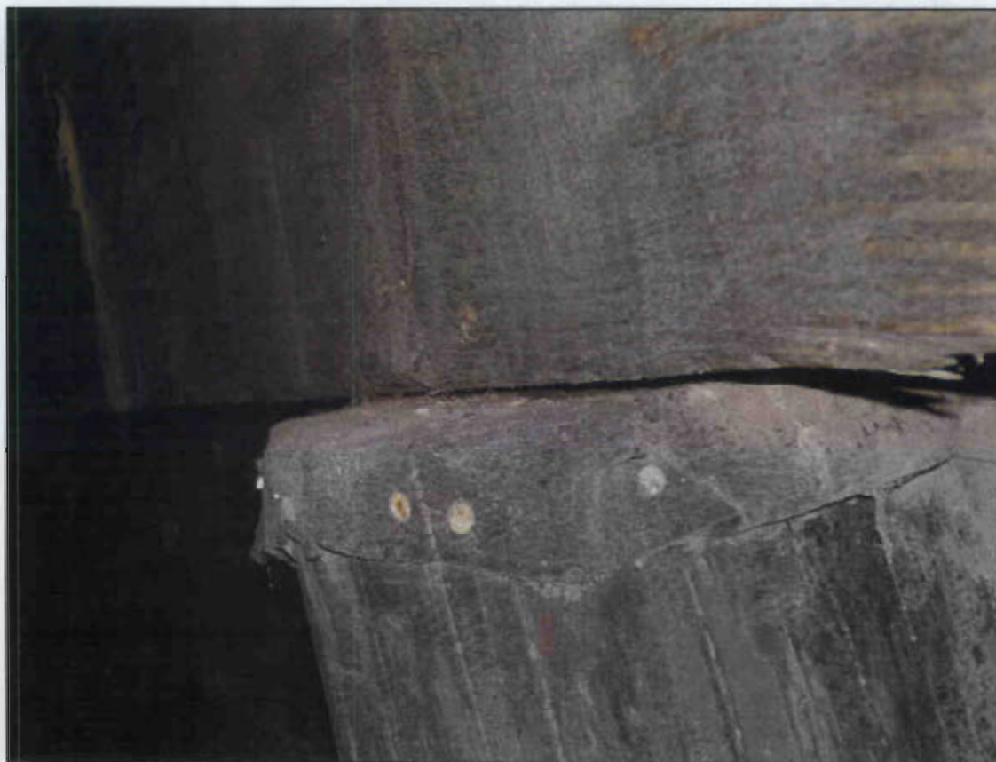
PILE 5 AT END BENT 2 PUSHED OUT 3" DUE TO BULKHEAD PRESSURE. (PRIORITY MAINTENANCE)
