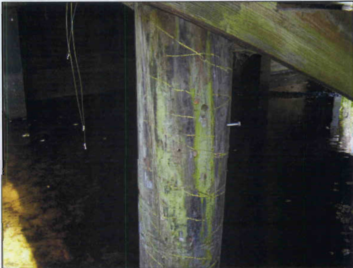
PILE 1 AT BENT 1 EAST SIDE DECAYED 32" HIGH X 6" DEEP X 1/2 CIRCUMFERENCE.(PRIORITY MAINTENANCE)
