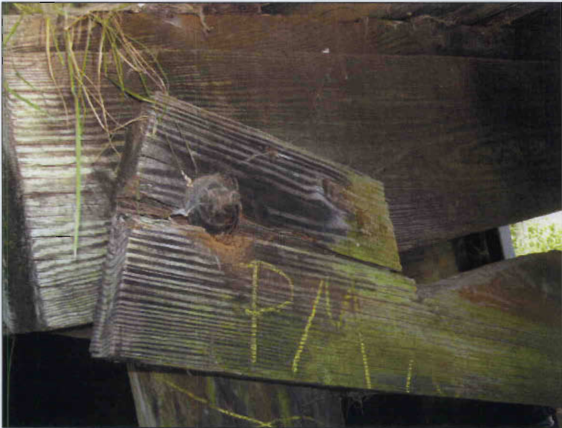
CROSSBRACE AT BENT 1 EAST SIDE AT PILE 4 SPLIT AT CONNECTION BOLT 1" WIDE X 15" LONG.
