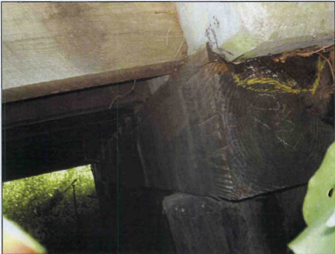
END BENT 2 CAP ROLLED BACK 1/4"
