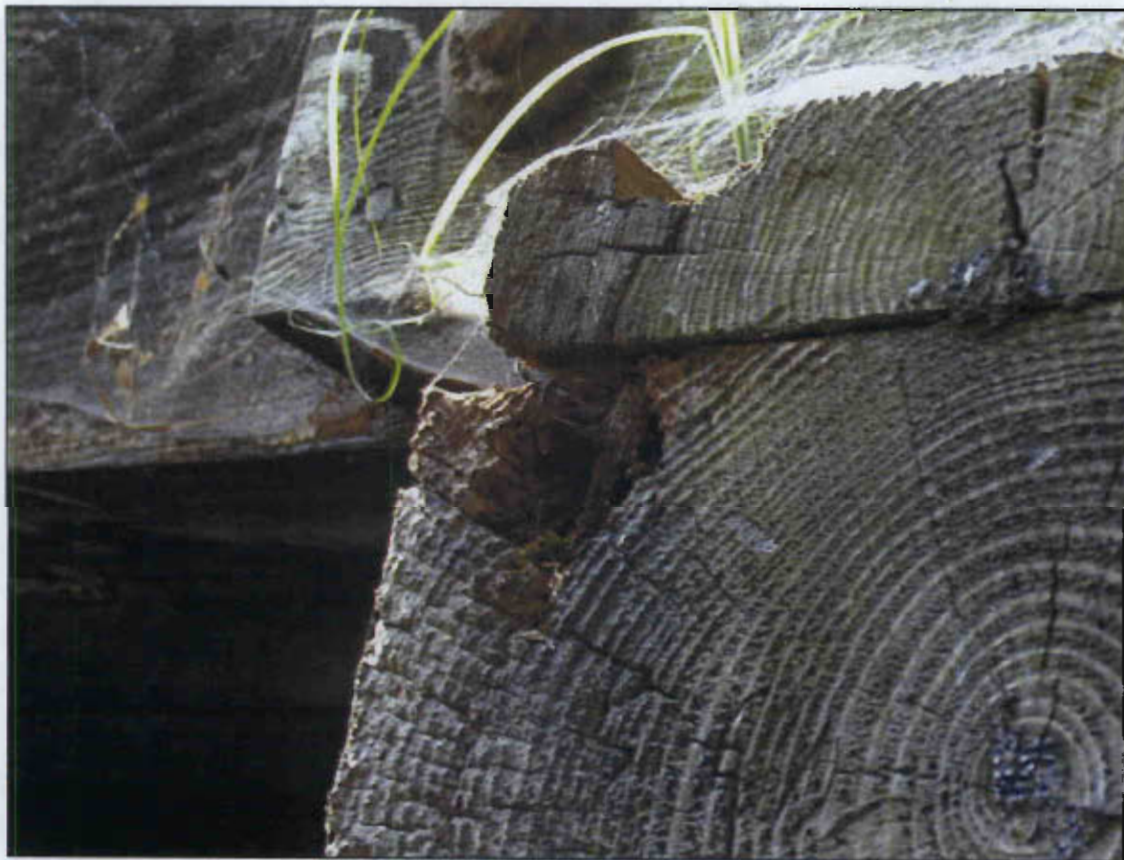
NORTH END OF BENT 2 CAP DECAYED AT TOP LEFT CORNER 3" DIA. X 3" DEEP.
