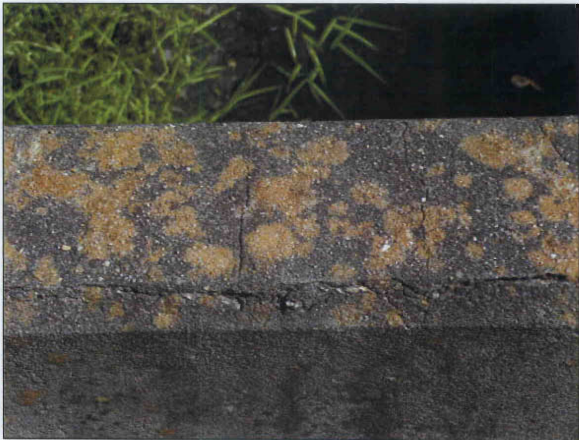
HORIZONTAL CRACKING ALONG NORTH RAIL BAR
