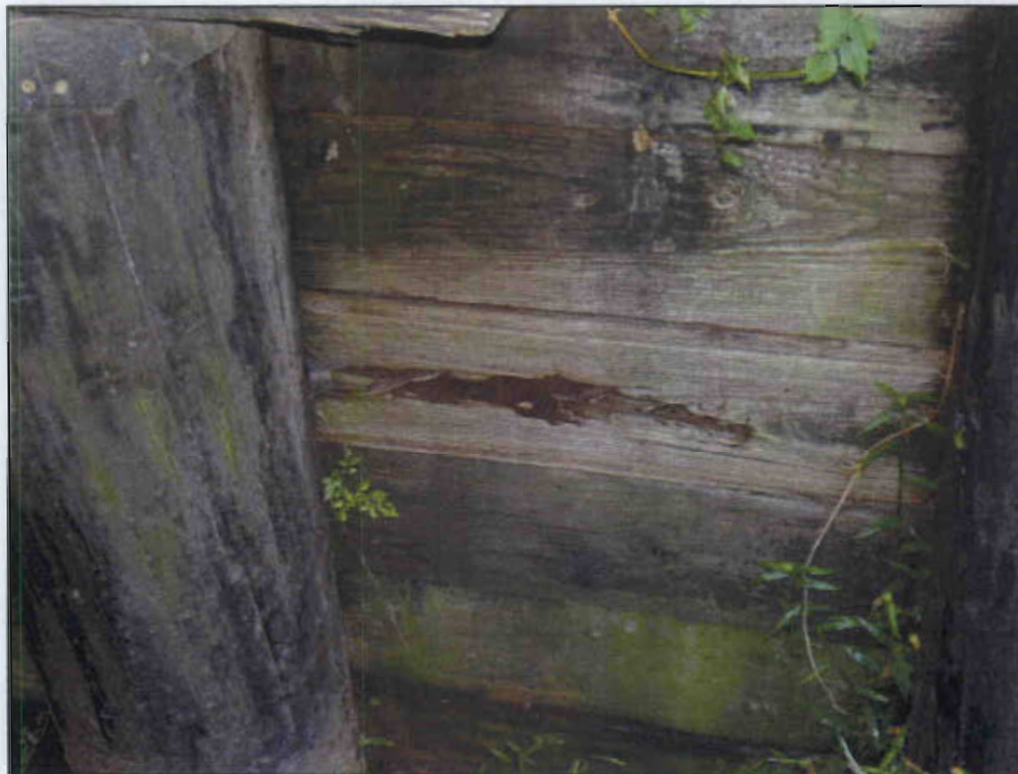
END BENT 2 BULKHEAD AT PILE 5 DECAYED AREA WITH EXPOSED FILL
