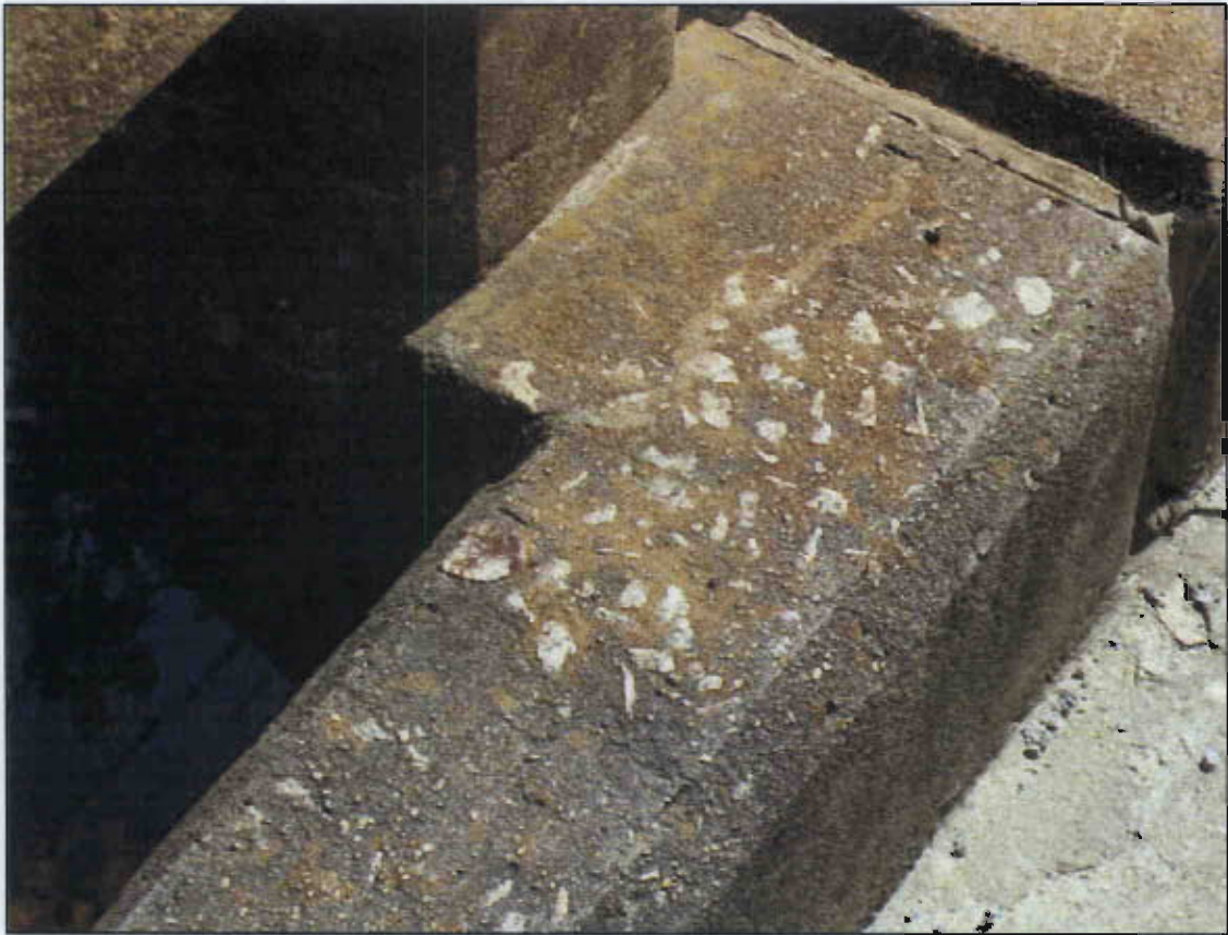
CURBS WEATHERED WITH EXPOSED AGGREGATE
