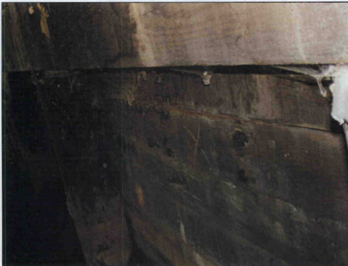
END BENT 2 BULKHEAD BOARDS PUSHED OUT UP TO 1"
