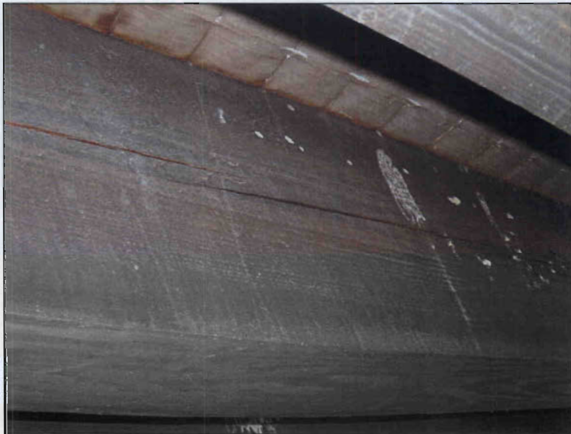
LONGITUDINAL CRACKING ALONG JOIST UP TO 1/8" WIDE.
