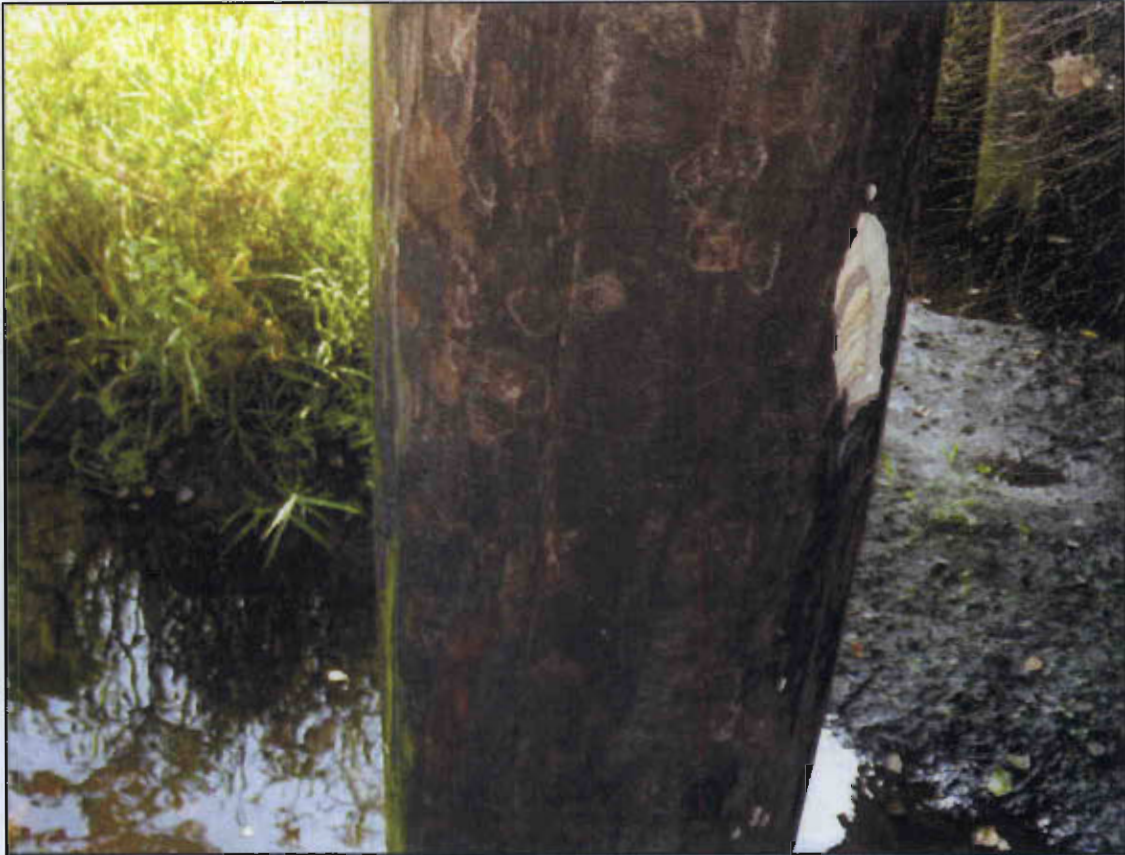
LONGITUDINAL CRACKING IN PILES UP TO 1/8" WIDE
