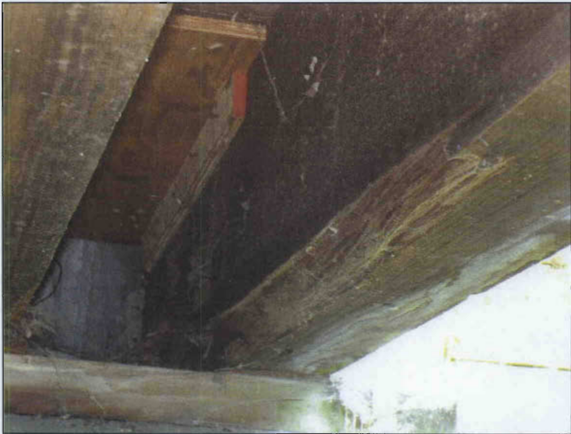
JOIST 1 IN SPAN 1 AT END BENT 1 SECTION LOSS 38" LONG X 2" WIDE X 2" HIGH
