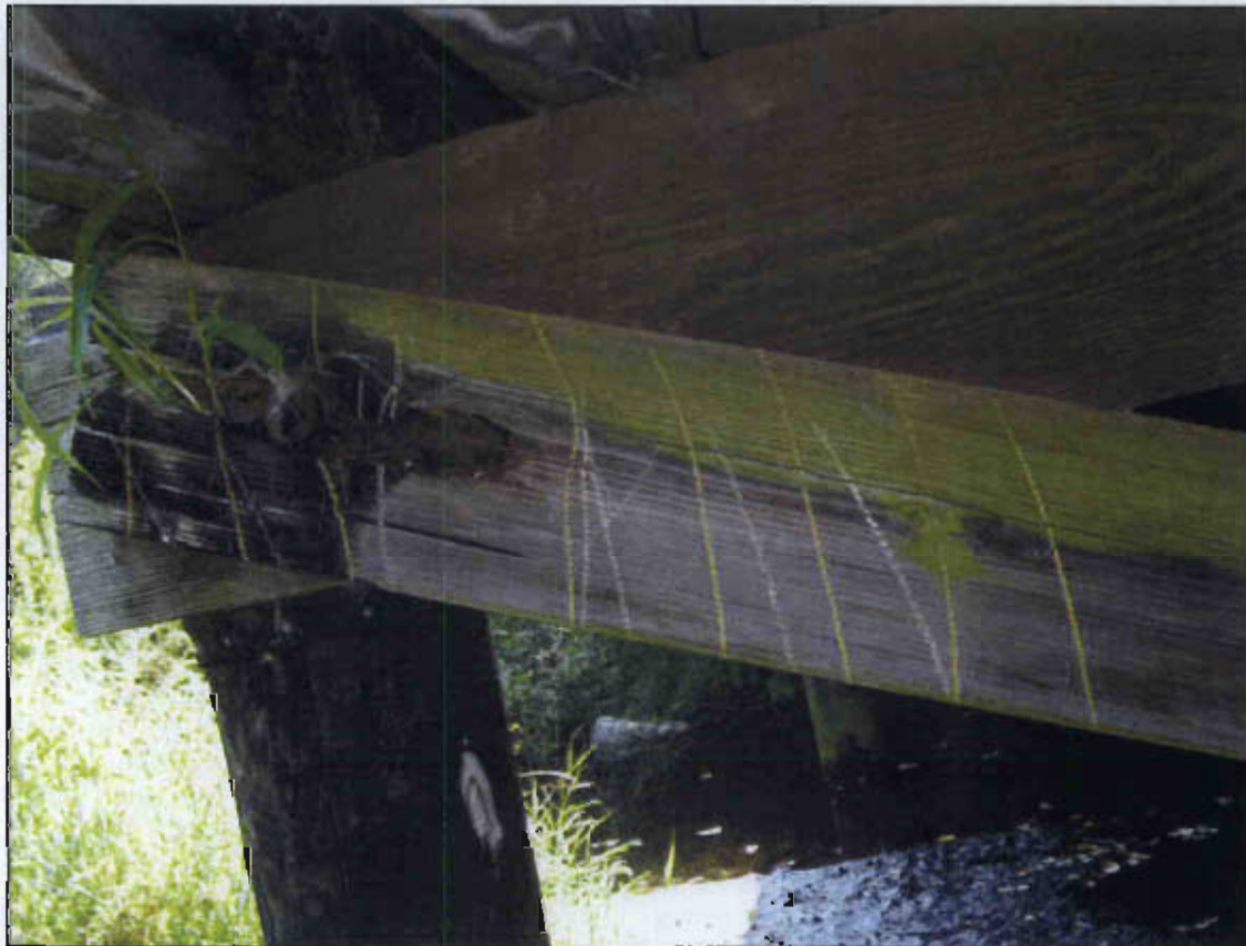
BENT 1 CROSSBRACE SPAN 1 SIDE AT PILE 1 DECAYED 4' LONG.
