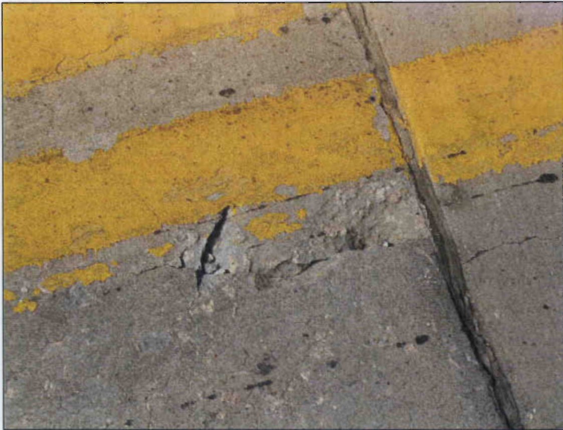
SPAN 3 DECK AT CENTERLINE ALONG BENT 2 CRACKED AND SPALLED AREA 4" WIDE X 12" LONG X 1" DEEP
