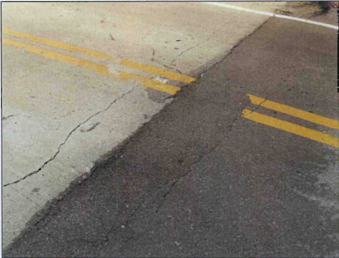
WEST APPROACH ASPHALT WEARING SURFACE CRACKED AND SETTLED UP TO 2"
